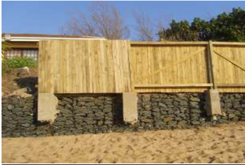
Plate 5.4: Preventative measures implemented for a beachfront property
