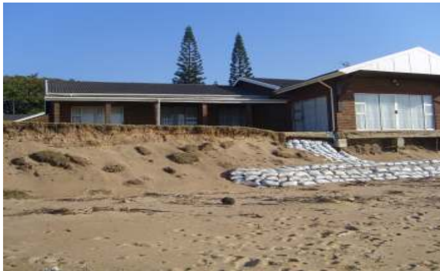
Plate 5.3: Damage to a beachfront properties, and the protective measures implemented
