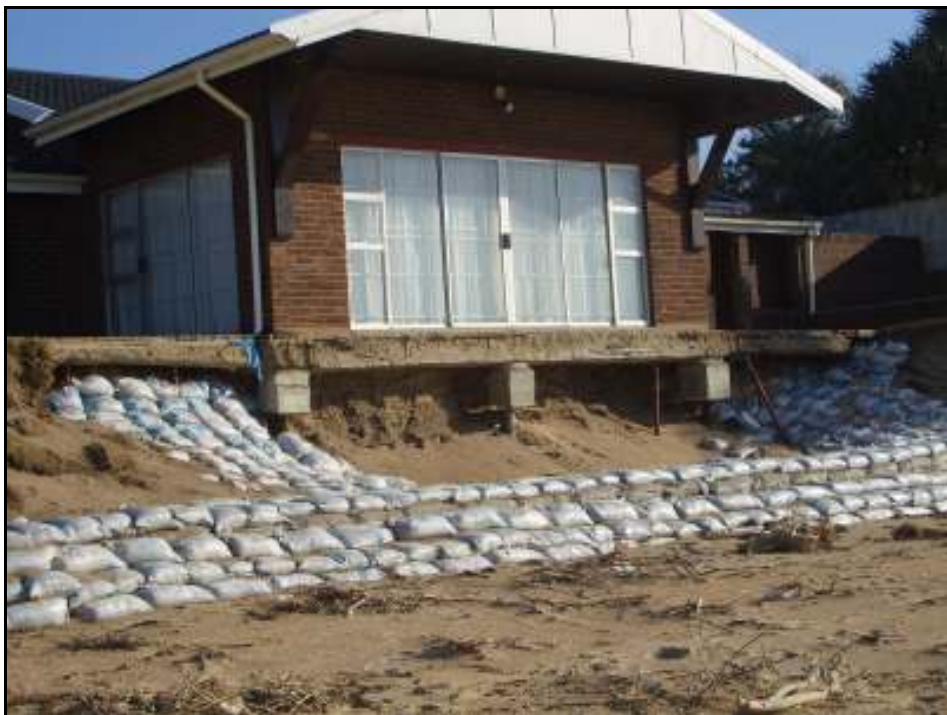
Figure 6: Damage to a property in Clansthal from recent storms, with sandbags to prevent further damage.
