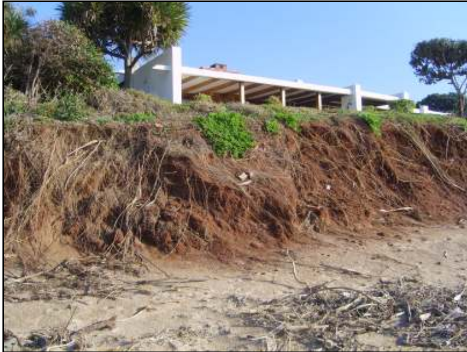
Figure 5: Wave damage to dune Vegetation.
